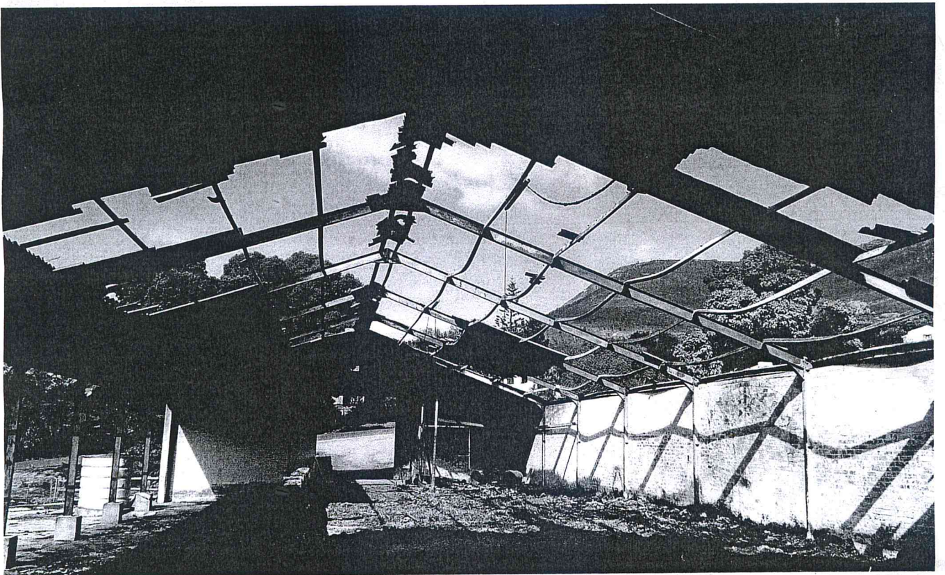
Damaged barn buildings after the fire
